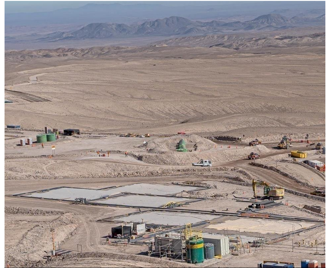
Image: View of site of new concentrator, with concrete foundations being laid and work to further prepare the site.
