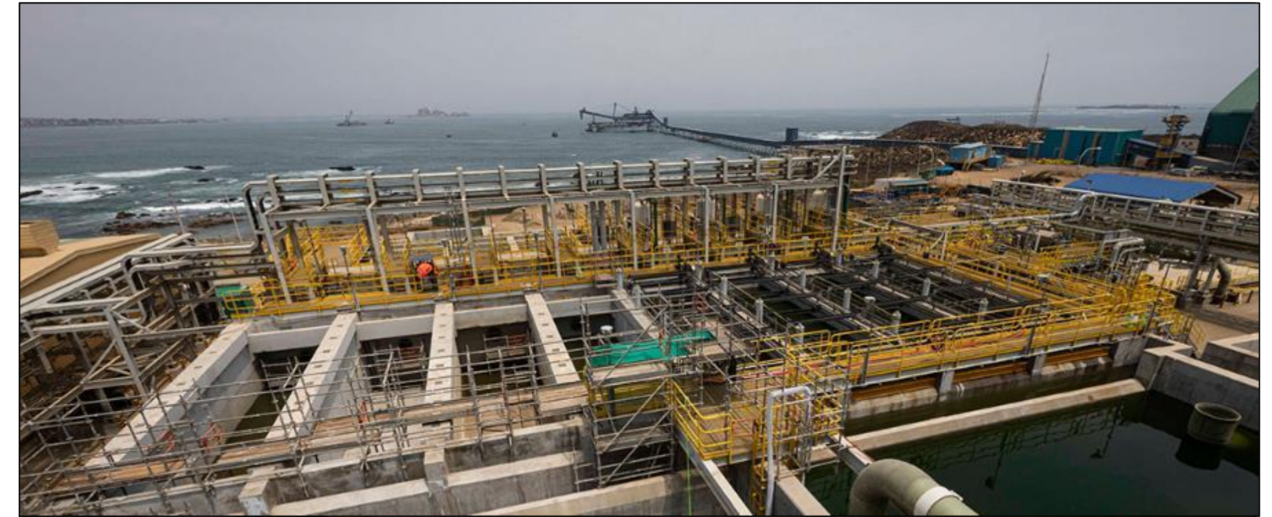
Image: Water tanks for existing desalination plant (right) and expansion (left)
